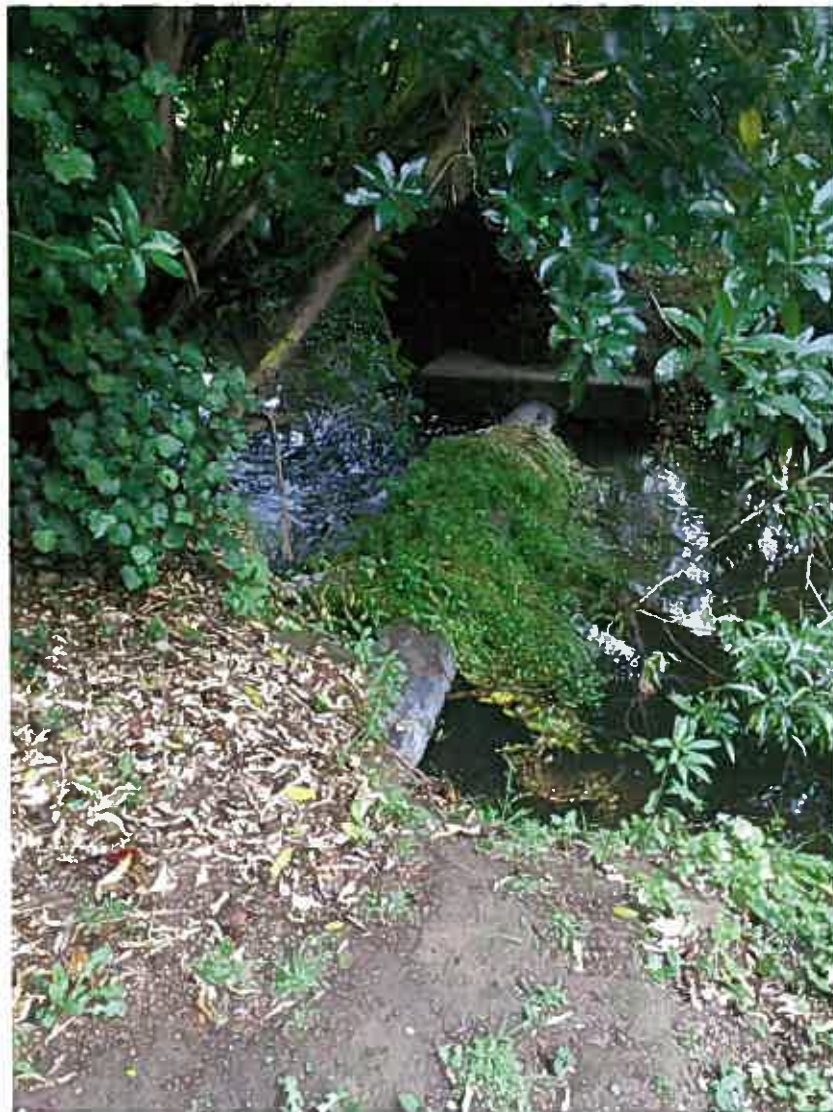
Photo 5 – Debris snagged on sewer pipe
