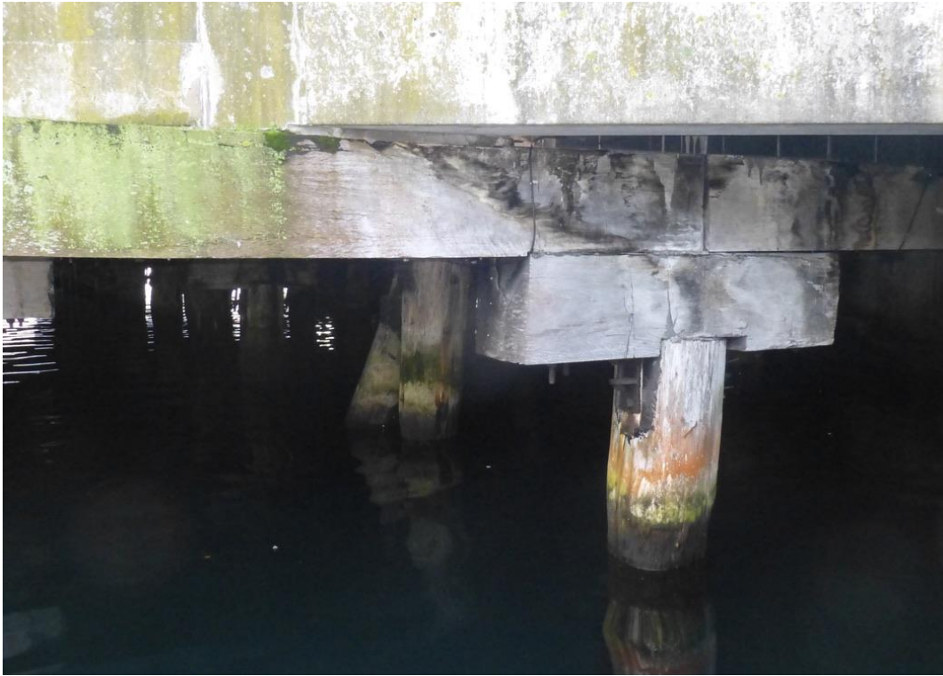
2 Piles, corbel and a major 400 x 400mm beam in the sub-deck structure of the breastwork.
