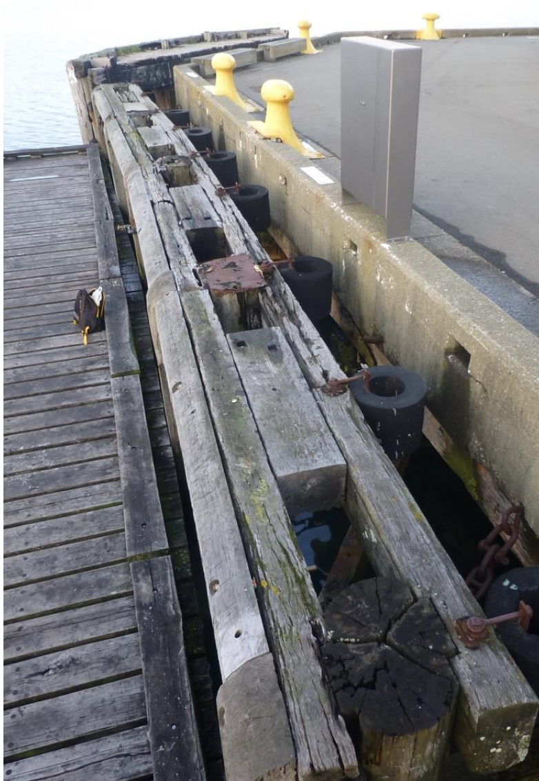
1 Heavy timber structure at the seaward end of the wharf, dating from the 1960s. Photo, June 2020.
