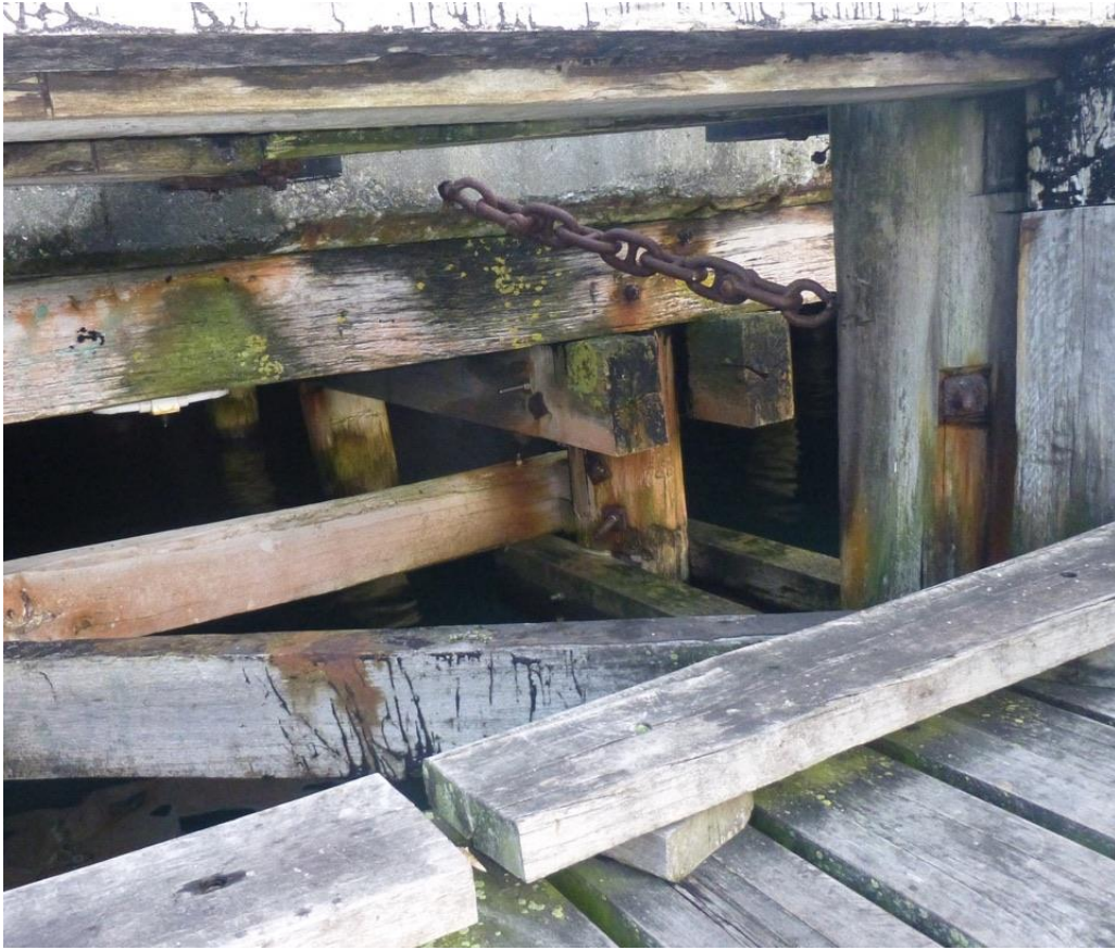
2 Detail of the structural timbers under the seaward end of the wharf. Photo, June 2020.
