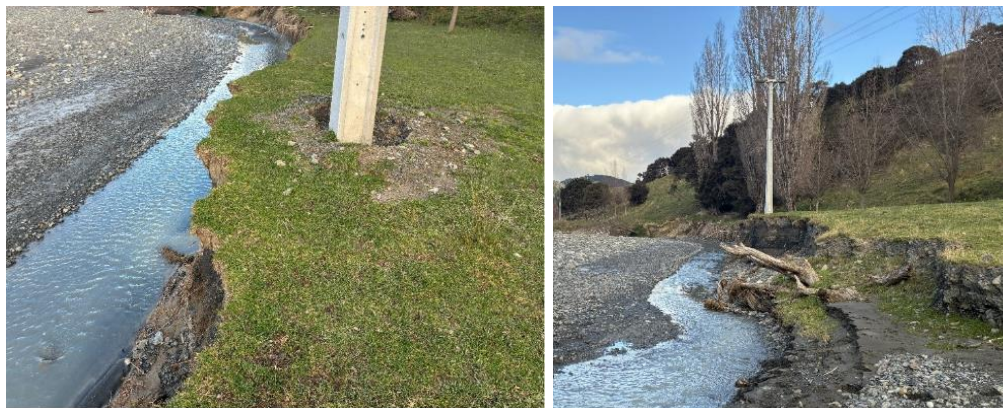
150. Image 20: Examples of some damage following the weather event.
