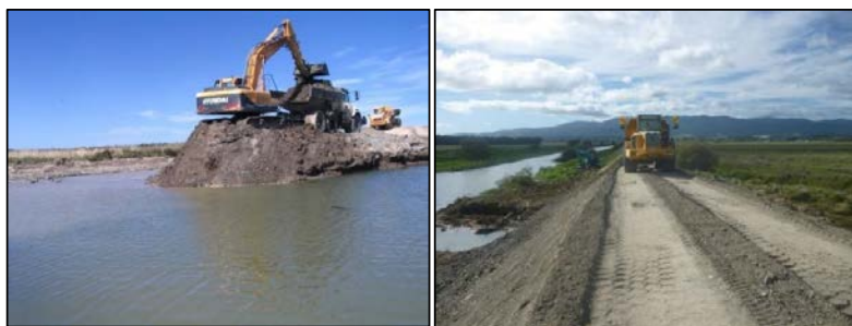
Ruamahanga River at Upland Cut Off Stopbank Before and After Damage (with Repair)
