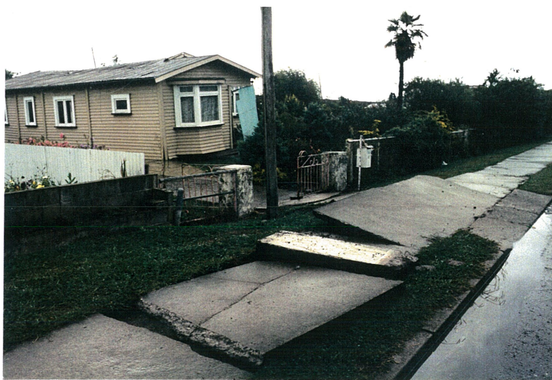
Photo 6. House thrown off its piles, south side of High Street Edgecumbe, note compression features in path.
