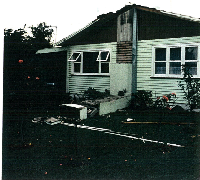
Photo 5. Chimney collapse, Kowhai Avenue, Edgecumbe.
