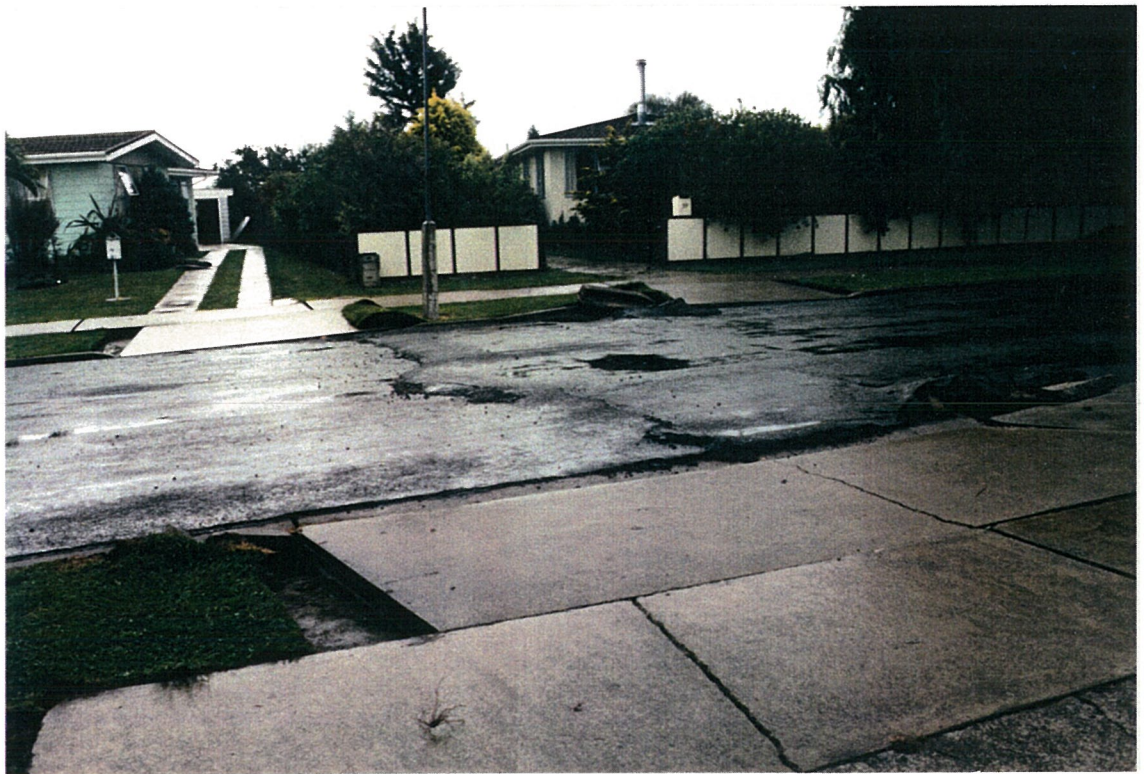
Photo 14. Compression flow in asphalt in Rata Avenue, Edgecumbe looking west, note north trending movement of pathway concrete blocks.
