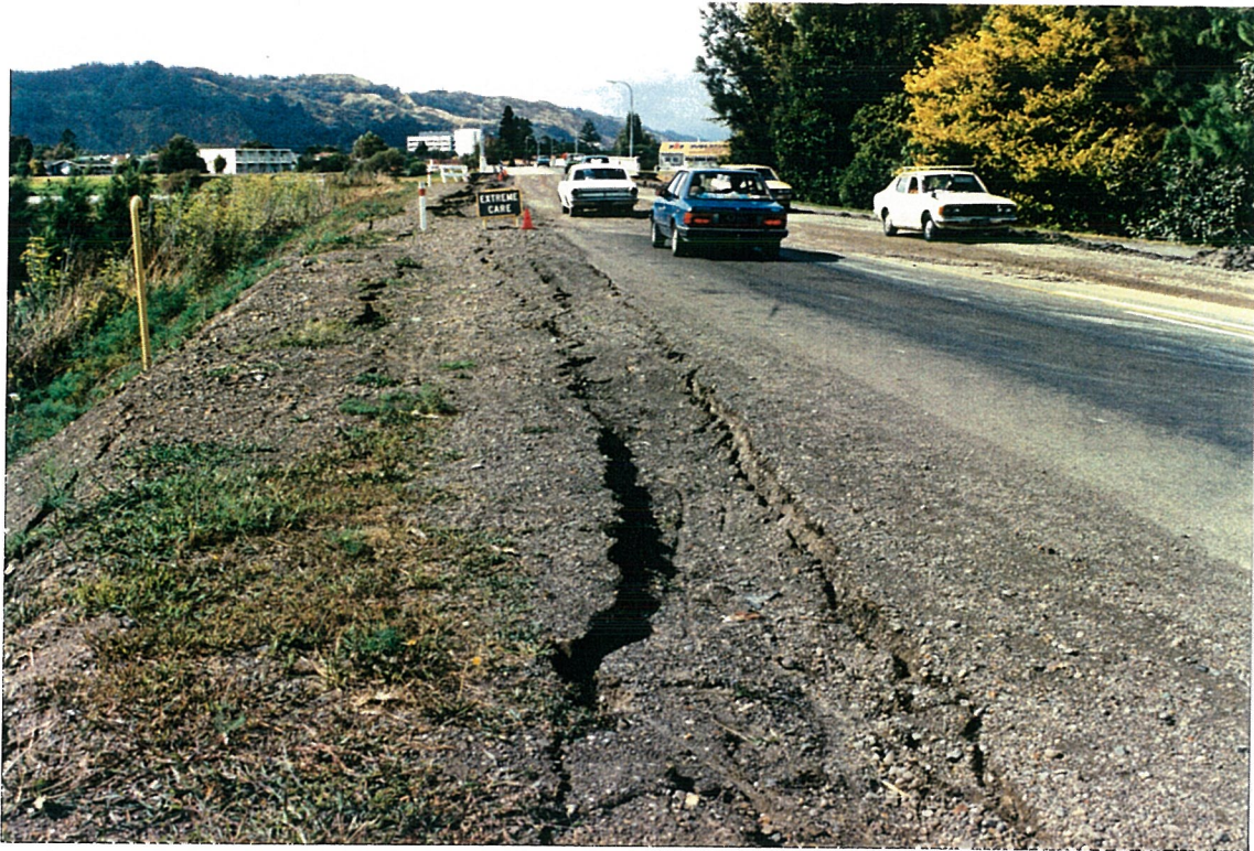
Photo 1. Settlement and spreading of the bridge abutment fill at Whakatane Bridge. With a duration of strong shaking of 8–9 seconds, the ground damage due to liquefaction effects was relatively slight. For a larger magnitude earthquake the duration of strong shaking would be longer (20–30 s for M 7.5, about 50 s for M 8) and the ground damage far more severe.
