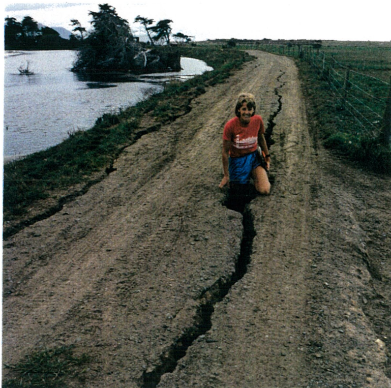
Photo 4. Lateral spreading and linear cracks on stop bank close to SH 2 at Greig Road.
