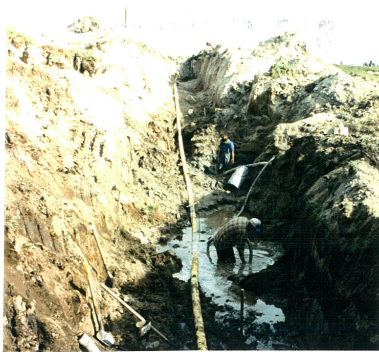
Photo 7. Excavation of high pressure gas pipeline through Edgecumbe fault, note sagging and distortion of pipe.
