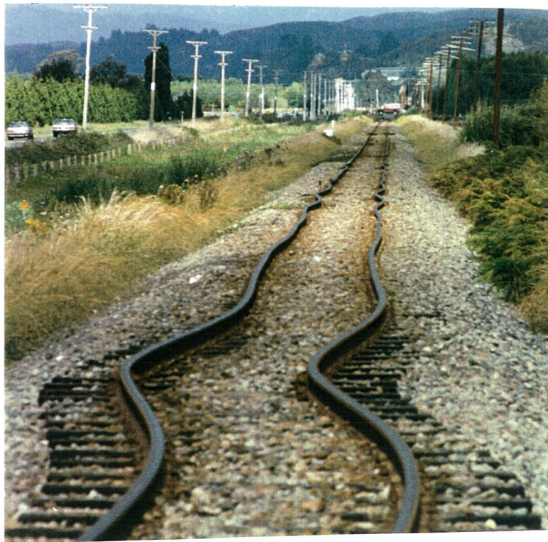
Photo 12. Compressional features in rail lines east of Edgecumbe.
