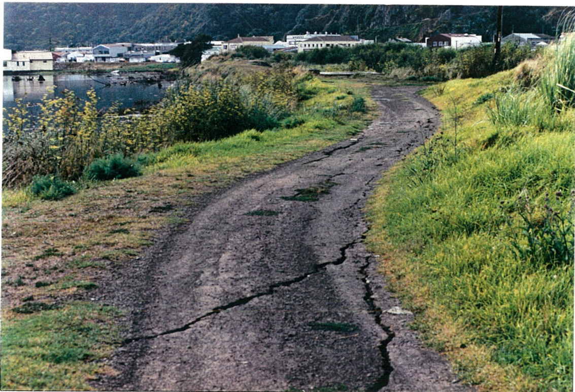
Photo 2. Fissures associated with lateral spreading in the river bank at Whakatane.
