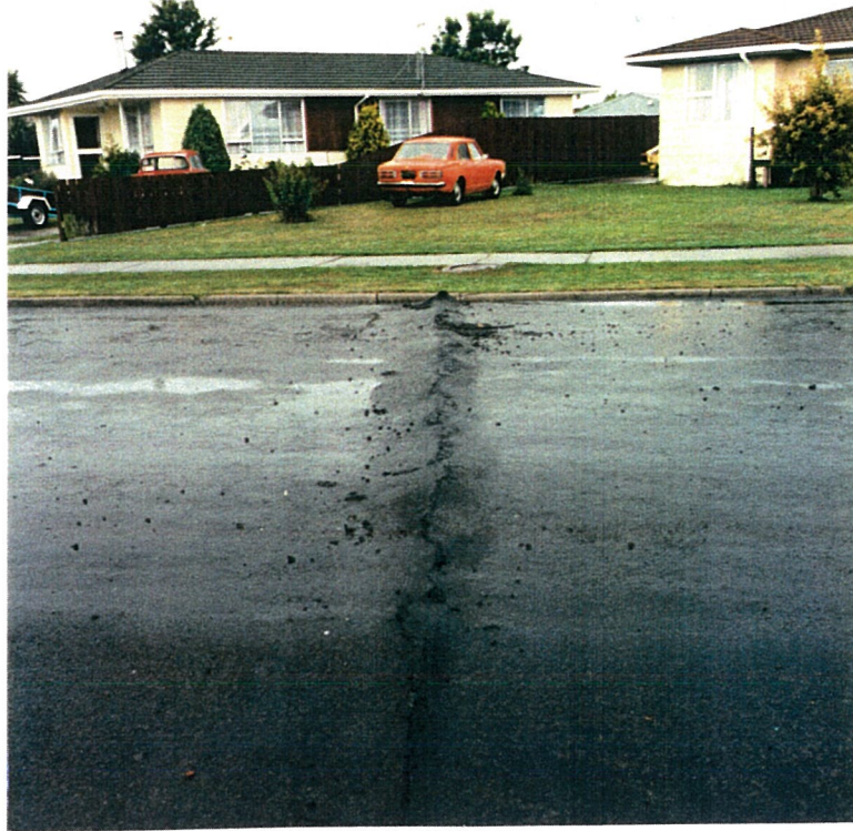
Photo 13. Compression ripple in asphalt surface of Rata Avenue, Edgecumbe.
