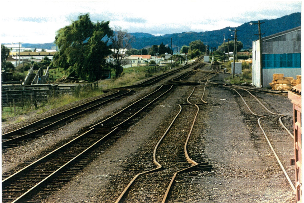
Photo 8. Railway lines damage at Edgecumbe station.
