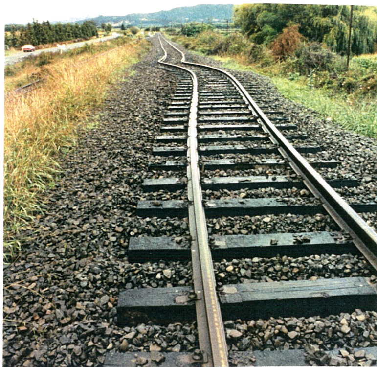
Photo 9. Railway sleepers 'vibrated' out of stone ballast on embankment opposite Bay Milk Company, Edgumbe.
