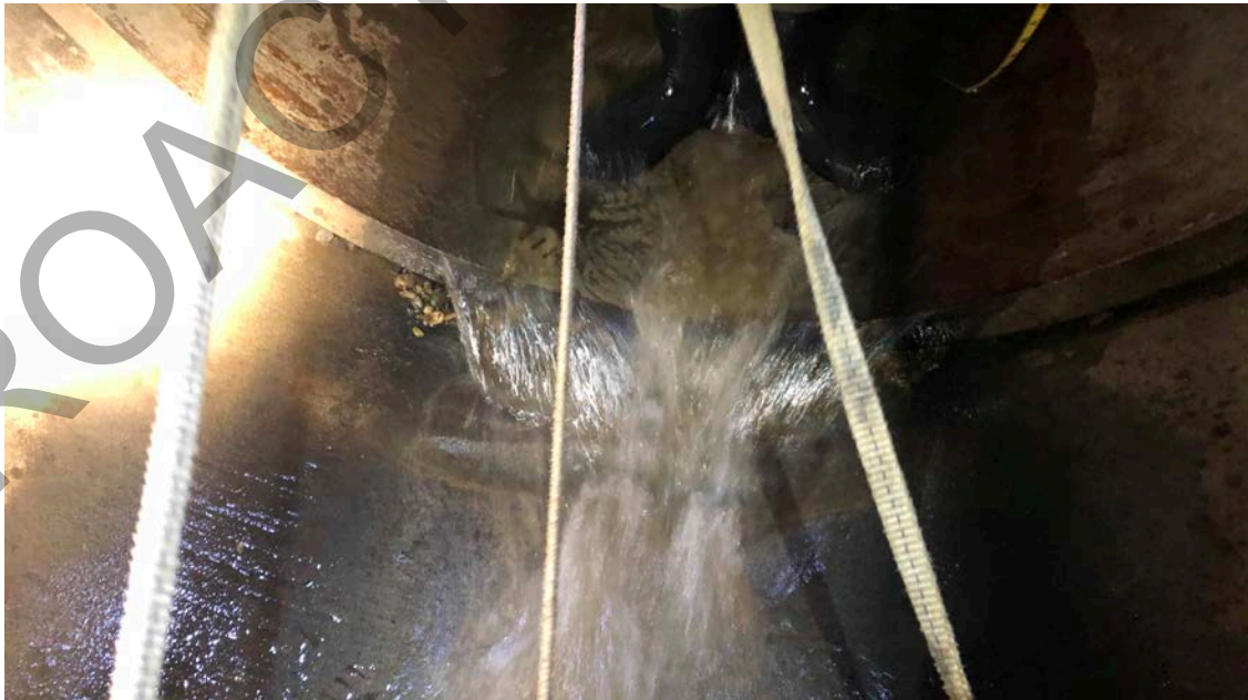
Figure 25 A change in circular, concrete pipe dimensions in Pae Kawakawa Stream under The Parade in Island Bay in a high velocity section of piped stream has created a small, undercut drop that may impede fish passage.
