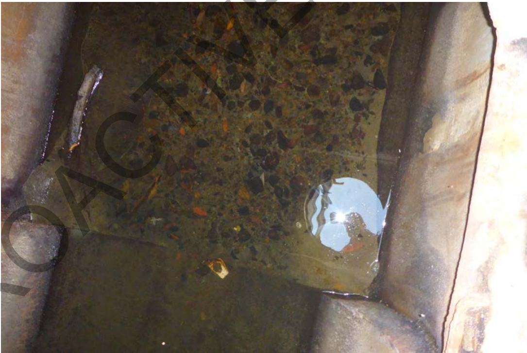
Figure 23 Pipe design at the Miramar Park site allowed the development of deeper pool-like habitat.
