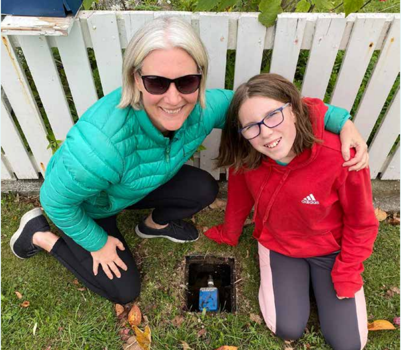
Gretchen Saulbrey (left) and her daughter Annalise Smith with their new smart water meter, installed as part of the Greytown Smart Meter Trial.
