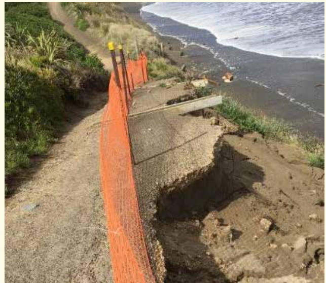
QEP coastal track after February 2018 storm. More frequent and severe storms as part of climate change means that the coastal track will progressively move inland where its less susceptible to damage.
