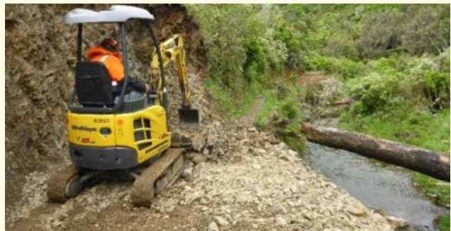
Flood damage repairs to the Korokoro Dam track provided the opportunity to improve the track and make it more resilient to future flood events.
