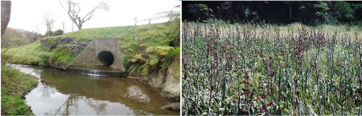
Perched culvert emptying into Kenepuru Stream (left) and Taupo swamp flaxland (right).
