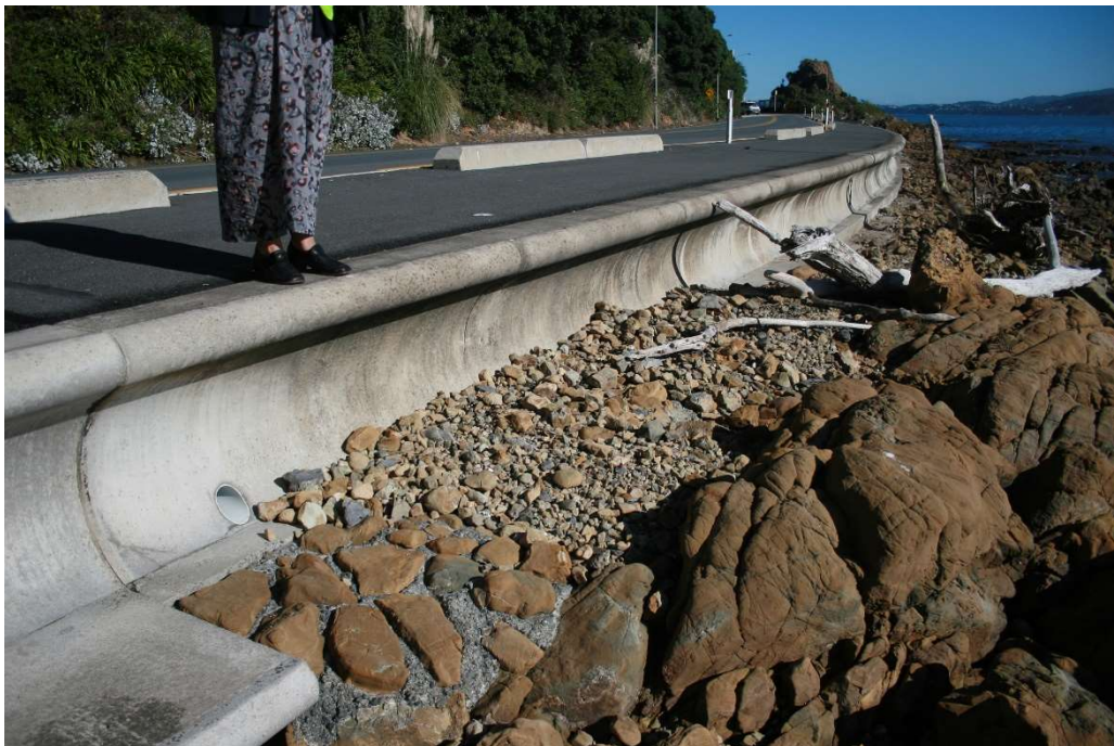
Figure 3 Unnatural transition from sea wall to rocky beach (to be avoided). The squared off end of the tread dominates the rock. It would have improved this transition if a large rock or a few large rocks were partially cast in to the end of the tread with minimal visible grouting (as opposed to here where the rocks set in the concrete matrix appears highly unnatural). Photograph by J. Head May 2, 2019.
