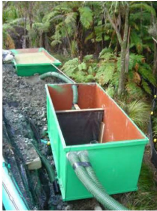
Figure 8.9.2.1: dewatering skip bin
