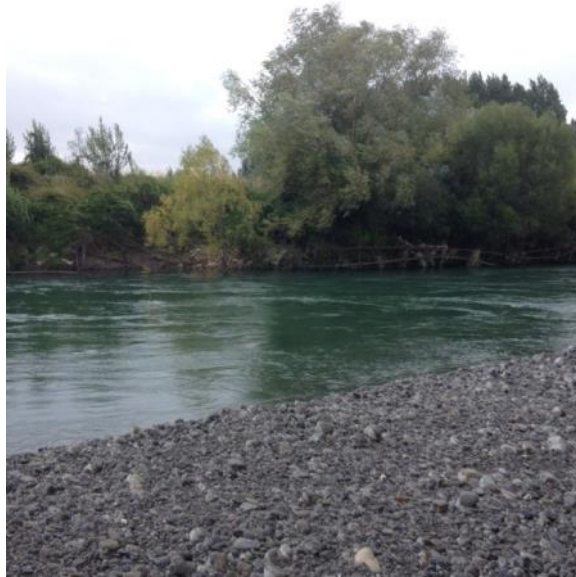
Waiohine River, Fullers Bend rightbank erosion – February 2017
