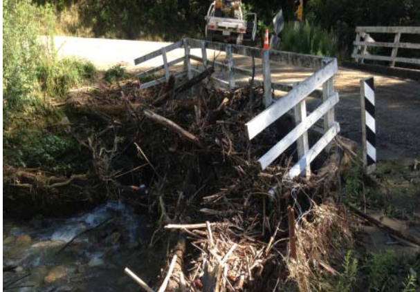
Debris blocking a local bridge
