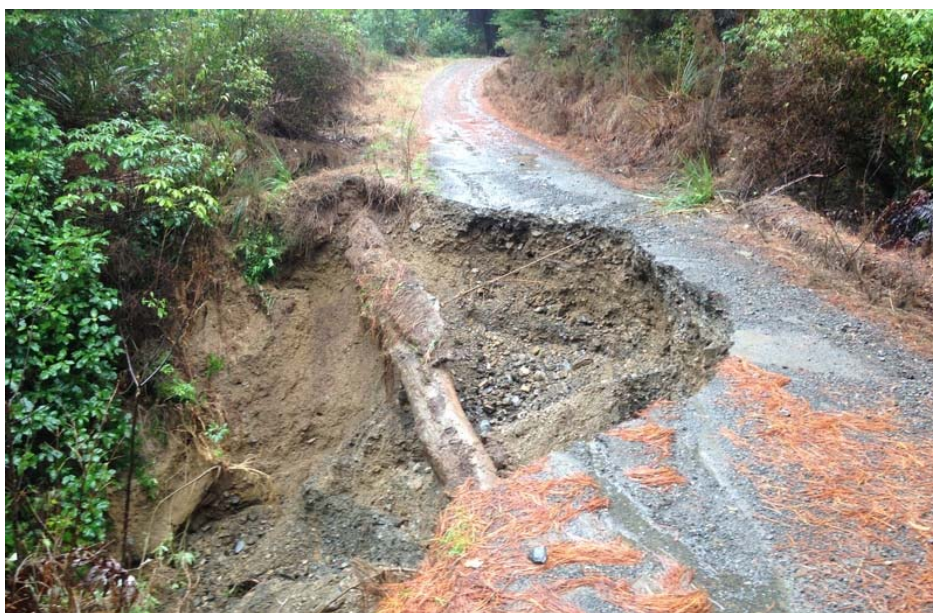
Subsidence on the Hukinga Road
