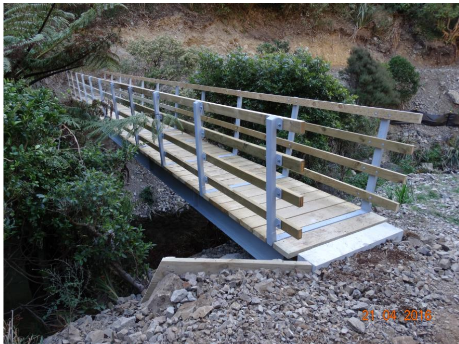
Helicopter installation of the new steel beam bridge at Korokoro (Belmont Regional Park).
