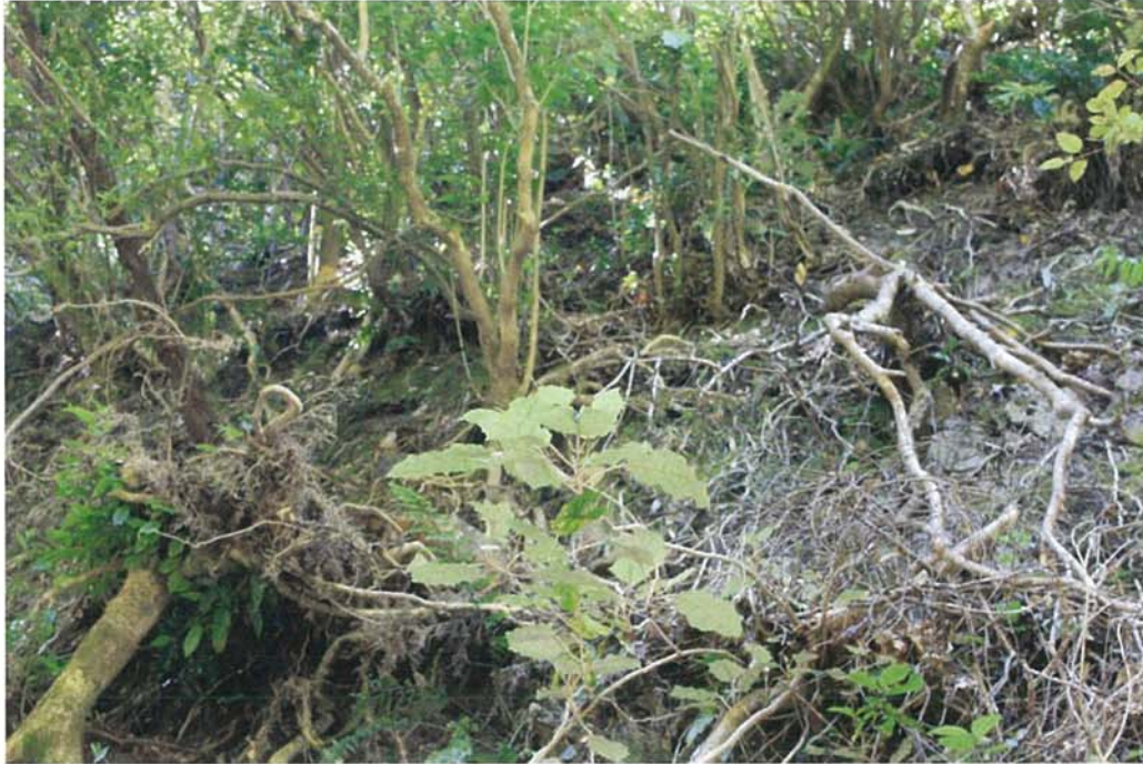
Figure 7: Above Ladle Bend, tree fall on batters on the Rail Trail cutting (Photo: Owen Spearpoint)
