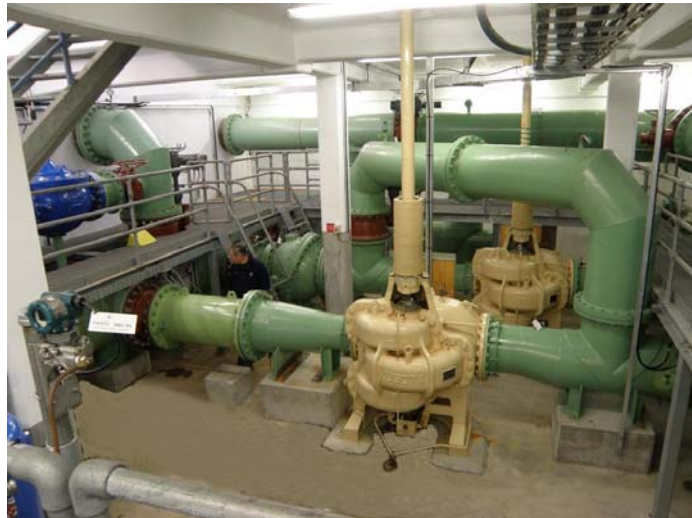
Figure 1 Te Marua lake pumps being used as turbines
