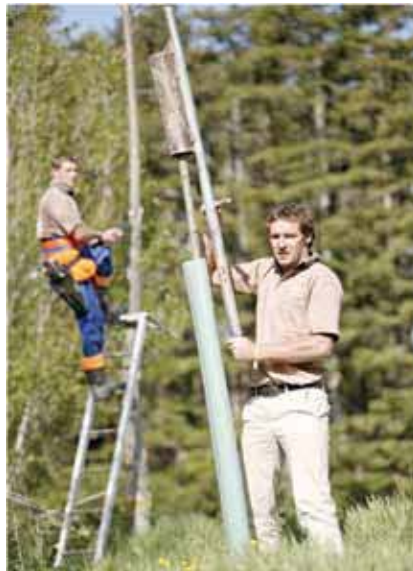
Planting poplar poles on erosion prone soils in the Wairarapa. Over 19,500 poplars were planted during 2008/09.
