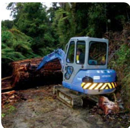
A rata had to be cleared from the Orongorongo access road
