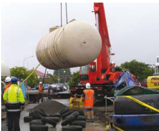
We have increased our diesel reserve at Waterloo following the installation of a new storage tank.
