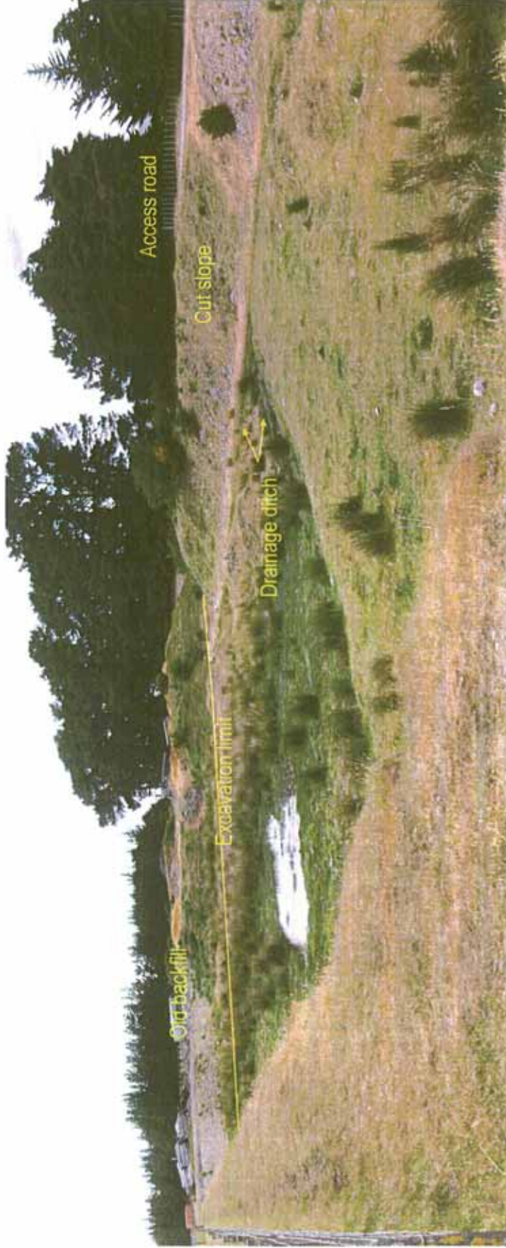
Figure 6. Eastern extension to old quarry excavation, partially backfilled with soil and inert fill. Looking south.
