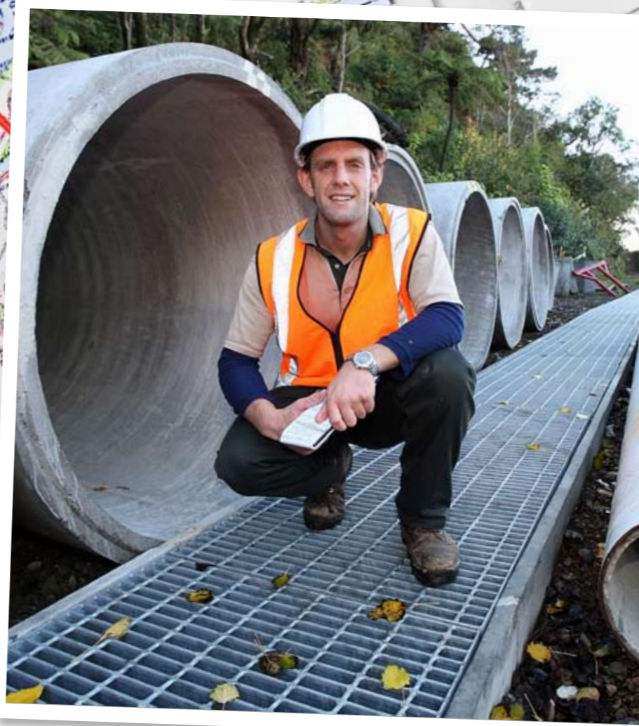
Above: Resource Adviser Jeremy Rusbatch on site at the Dowse-to-Petone roadworks. Centre: Back at the office, poring over plans for a proposed subdivision with fellow resource adviser Tyro Baker-Underhill. Left: Jeremy assesses earthworks near the Petone-Dowse flyover
