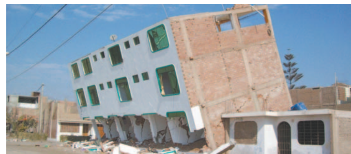
Building on a lean after the Peru earthquake, August 2007. Photo courtesy of Dr David Hopkins (David Hopkins Consulting Limited)
