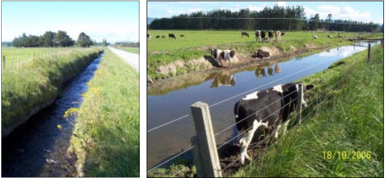
Figure 6: Battersea Drain at Fenwicks Line. Left – shows the straight, open channel. Right – near the confluence with Otukura Stream there is stock access and eroding banks.
