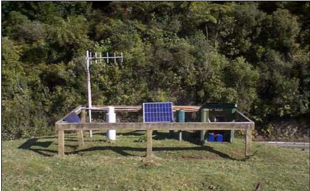
Figure 7: Transmission Lines rainfall station
